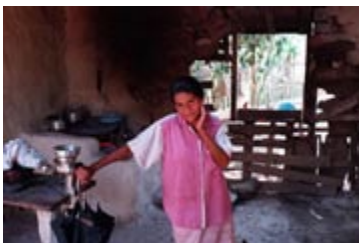
Hurricane Mitch damaged the walls of Guadalupe Barrientos' home (rear) in San Jose, and
